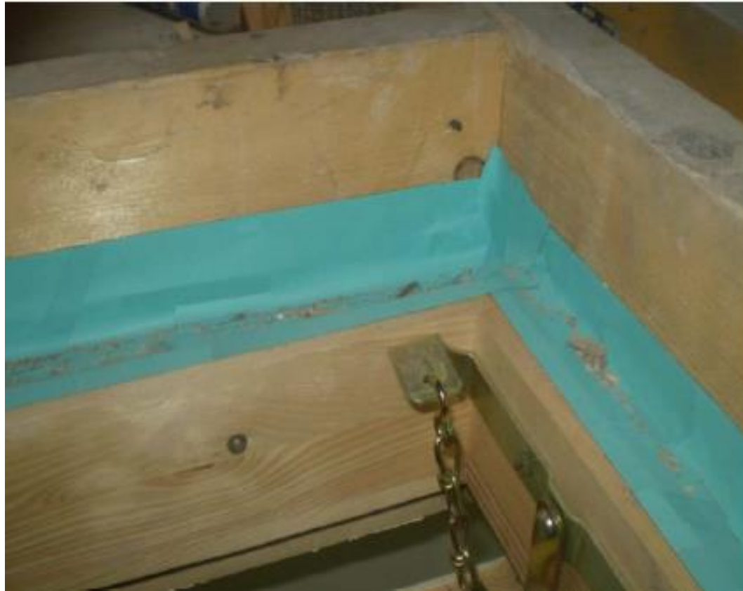
Sealing around frame of access hatch to attic
