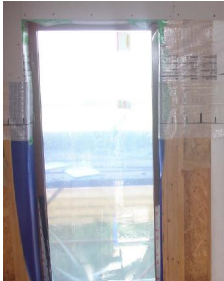
Sealing under way at junction of timber frame wall and external wall ope
